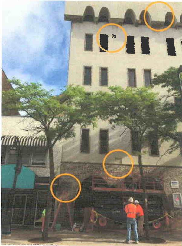
Locations of some of the probes on the State Street Façade. August 20, 2015.
