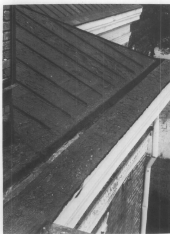
Repeated repair with asphalt, which cracks as it hardens, has created a blistered surface on this sheet-metal roof and built-in gutter, which will retain water. Repairs could be made by carefully heating and scraping the surface clean, repairing the holes in the metal with a flexible mastic compound or a metal patch, and coating the surface with a fibre paint. (Roane County Courthouse, Kingston, Tennessee, photo courtesy of Building Conservation Technology, Inc.)
