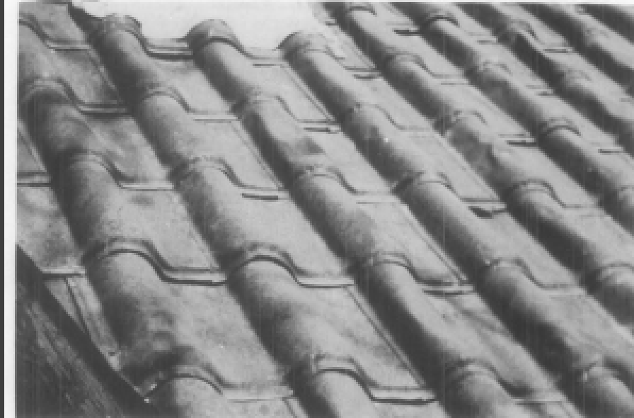
Galvanized sheet-metal shingles imitating the appearance of pantiles remained popular from the second half of the 19th century into the 20th century. (Episcopal Church, now the Jerome Historical Society Building, Jerome, Arizona, 1927)
