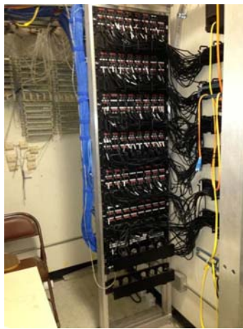
Figure 46 -- Third Floor Telecommunications
