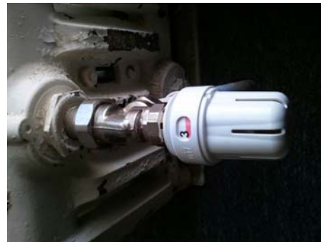
Figure 36 – Steam Radiator Control Valve
