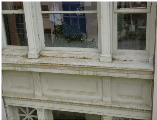
Figure 24 – Rust is Developing at Window Sills
