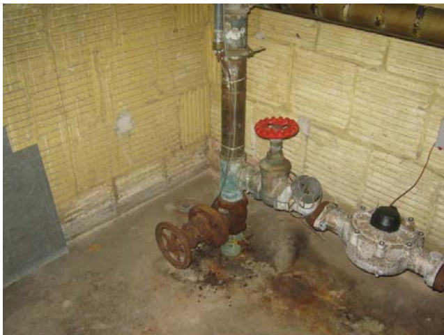
Figure 39 – Incoming Combined Plumbing and Fire Protection Service
