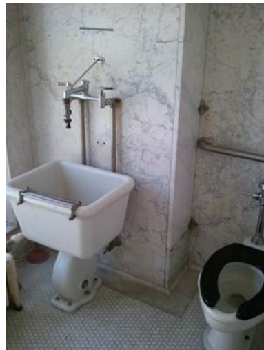
Figure 42 – Antiquated Plumbing Fixtures
