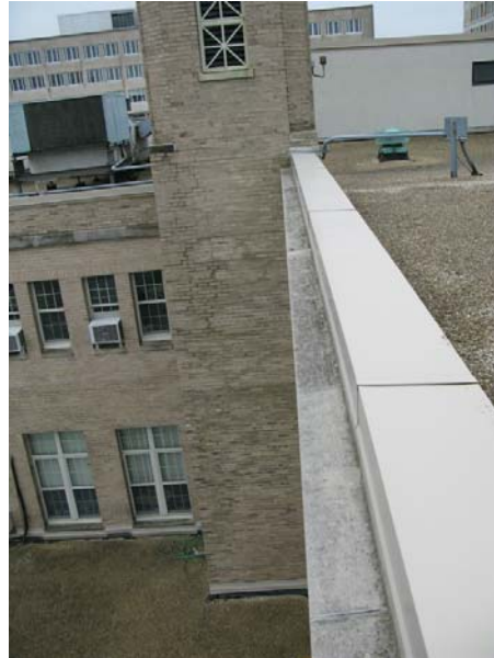
Figure 23 – Outside Corner of the Brick Chimney is Cracking Vertically on Both Sides
