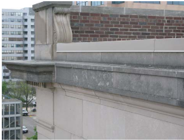
Figure 21 – Darkening of the Stone below the Metal Coping indicates Water Saturation
