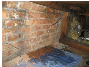
Figure 19 – Water Infiltration is occurring at the Raised Wood Roof Level.
