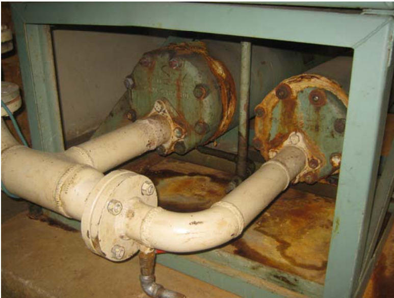
Figure 30 – Rust and Age Degradation on Heat Reclaim Chiller
