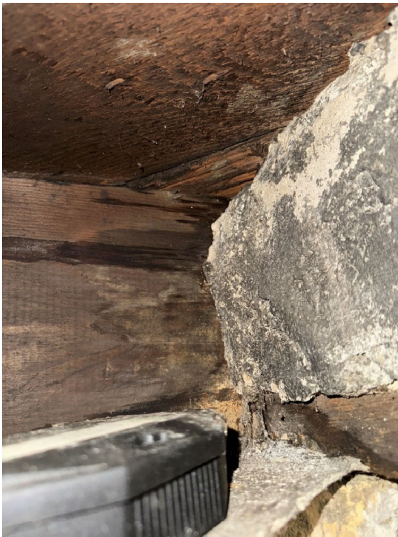
Bearing Floor Condition
