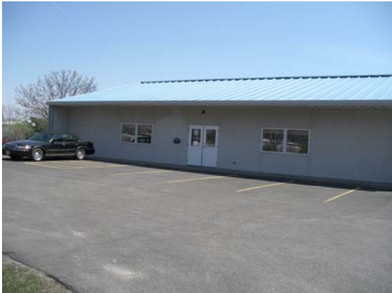
Parking lot lacks appropriate accessible parking signage for parking lot and restriping the entire parking lot will allow for a van access aisle. Depending on where the restriping lands, the cement pad in the front entrance may need to be adjusted to allow for ramp access.
