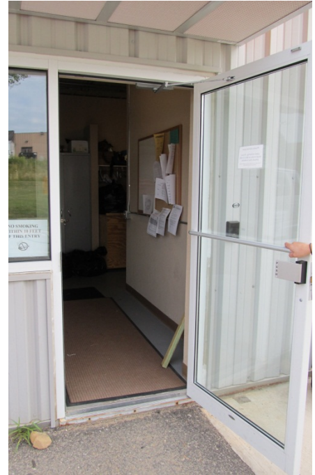
Side Entrance lacks power assist and the step needs to be removed to allow for wheel chair access. Improvements will level out concrete pad.
