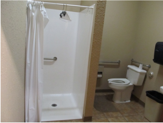
Shower does not allow for appropriate turn radius.
