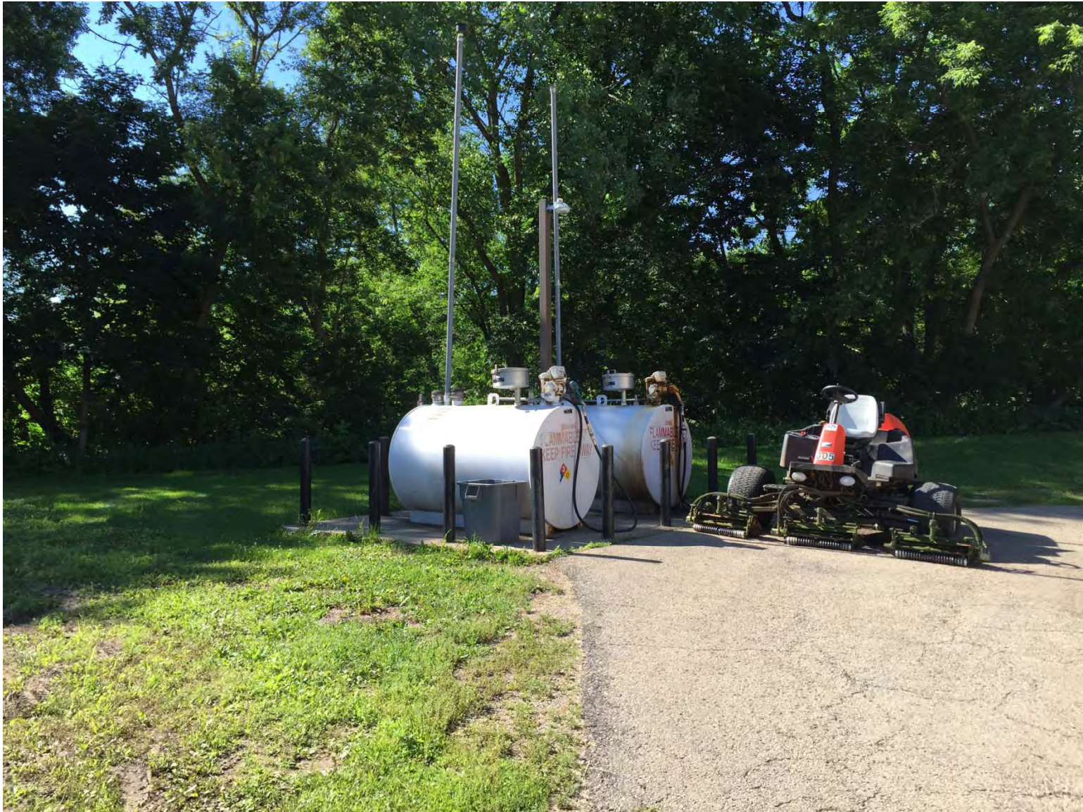
Forest Hill Yard M-6 : Fuel Dispensing Station
