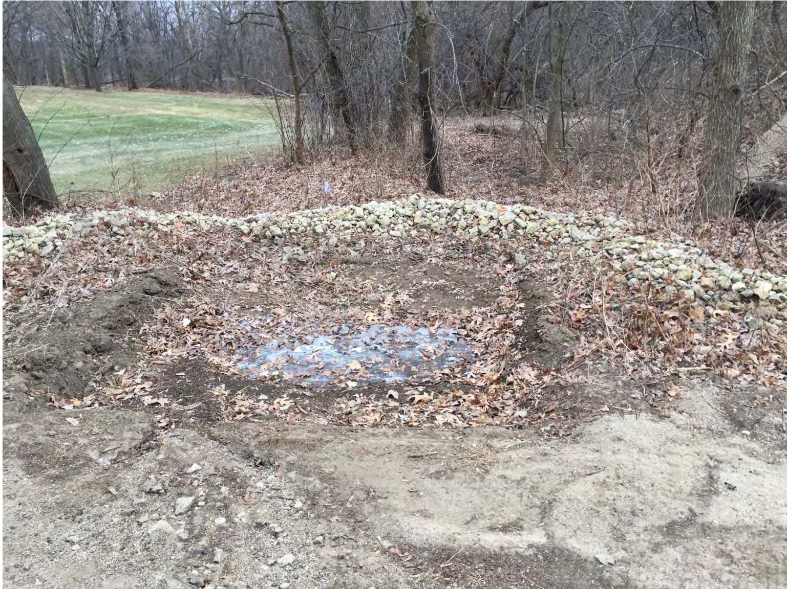
Forest Hill Yard M-7 : Stone Weeper Before Drainage Way
