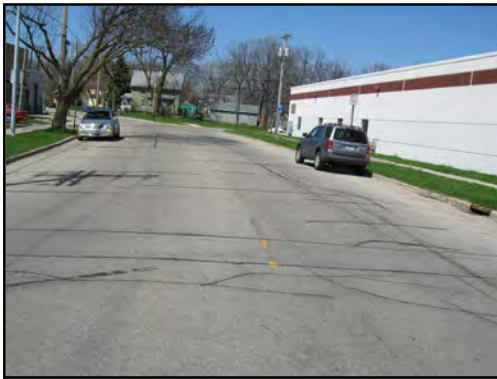
Beld Street (near Wingra), looking north (fairly good condition with tarred cracks)
