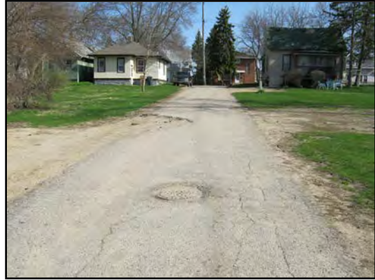
Garden Street, looking north (no sidewalks or curbs, cracks, & missing asphalt due to severe deterioration)
