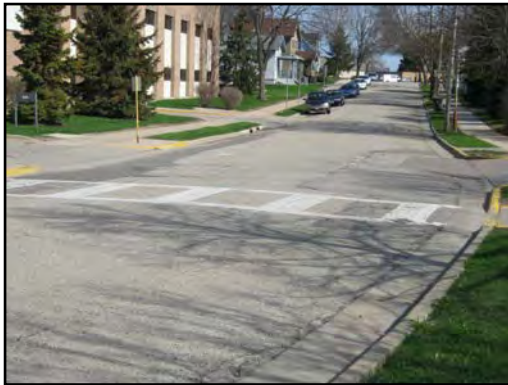
South Street (north of Appleton), looking north (patchwork, cracks, faded crosswalk striping)
