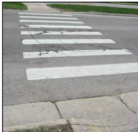
Park and Cedar, looking east (asphalt cracking, concrete curb cracking)
