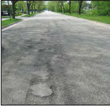
Plaenert (just west of Park), looking west (asphalt in fair to poor condition-crumbling)
