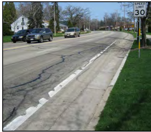
Fish Hatchery and Plaenert, looking north (cracks, tarred cracks, minor crumbling)
