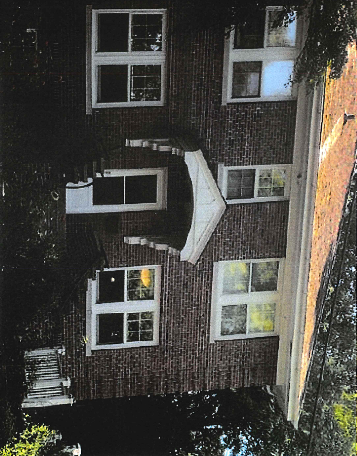
Upper Windows Recently Replaced Lower Mull Units to Be Replaced
